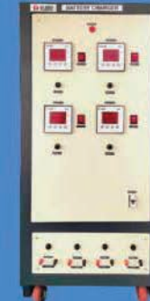
VRLA BATTERY CHARGER
